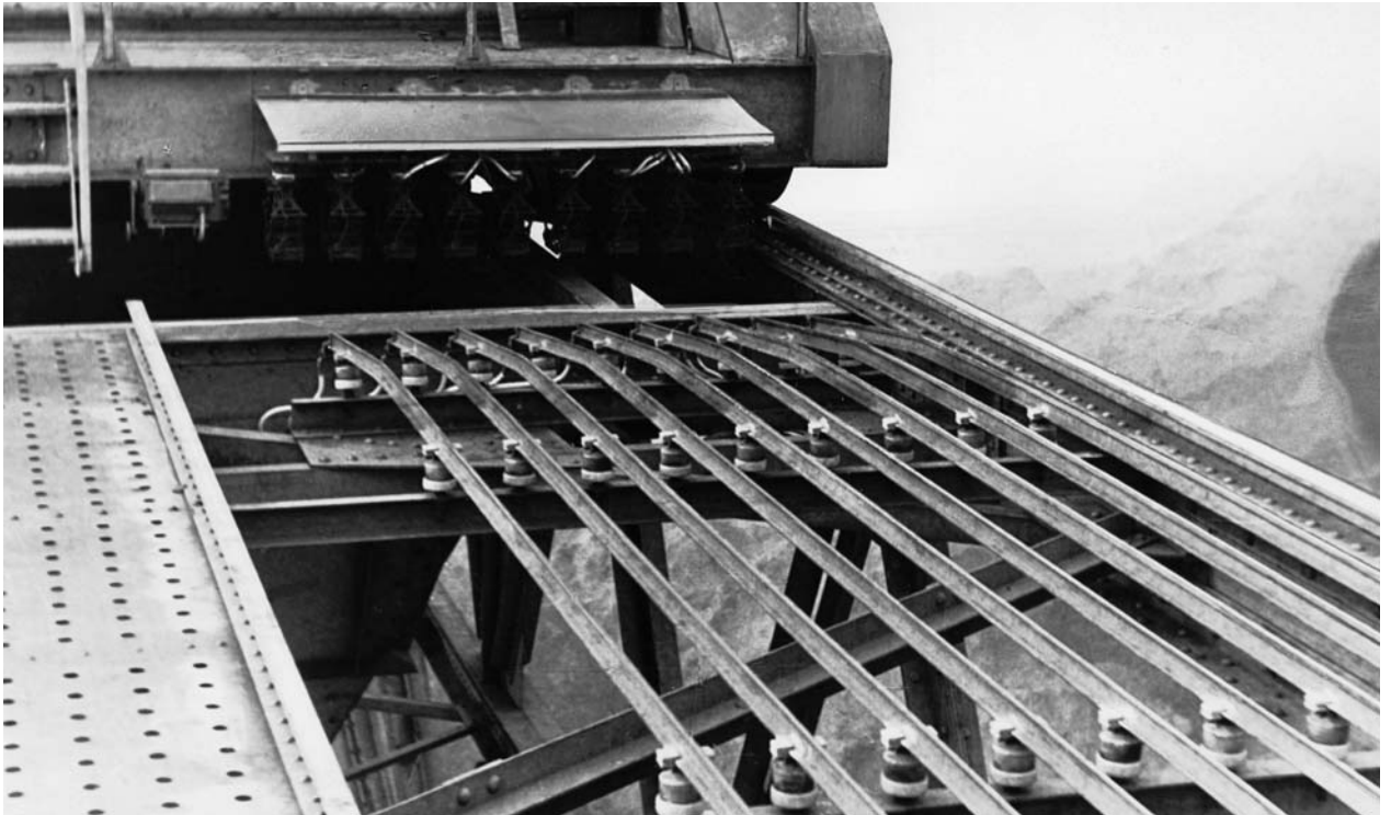
Bridge Crane Conductor Transfer Ends
